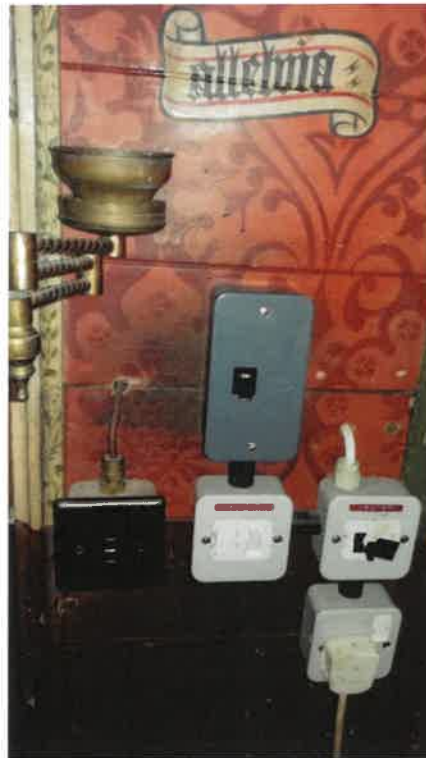
Variety of electrical fittings screwed into decorated case
