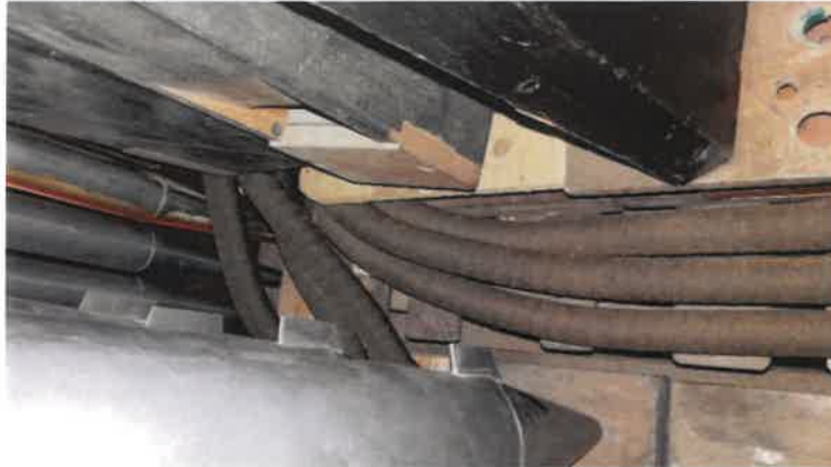
Flexible cardboard tubing to façade pipes
